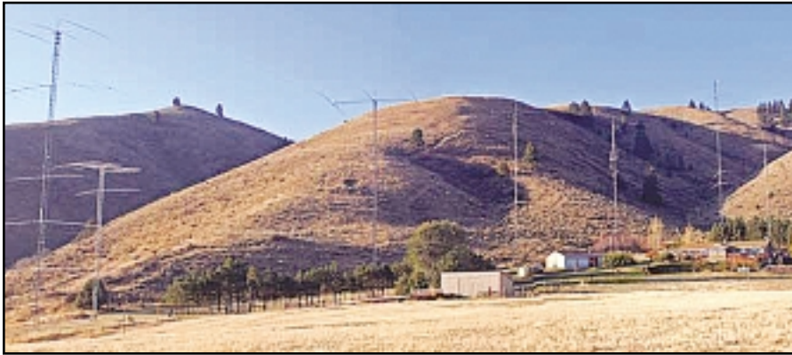
The antenna farm at NK7U, Multi-Single from eastern Oregon.
